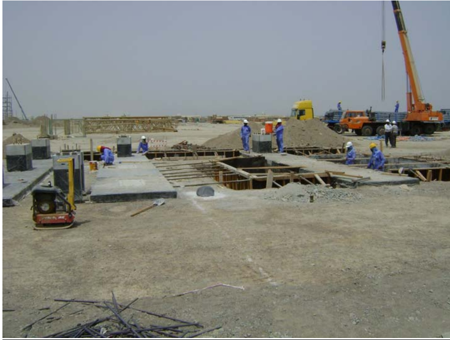
Fig. 11: Transfer Tower, TT-03
