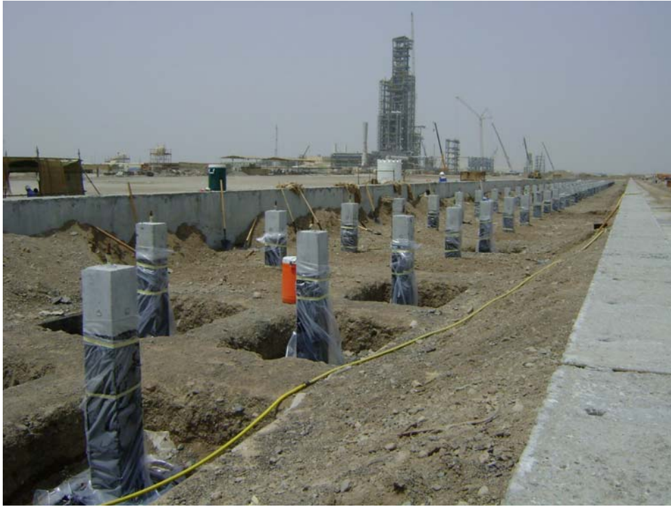
Fig. 9: Pedestal of Conveyor no. BC-03
