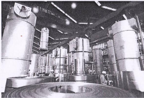
The hydrogen-based bell annealing furnace of Bhushan Power & Steel company at Sahibabad
